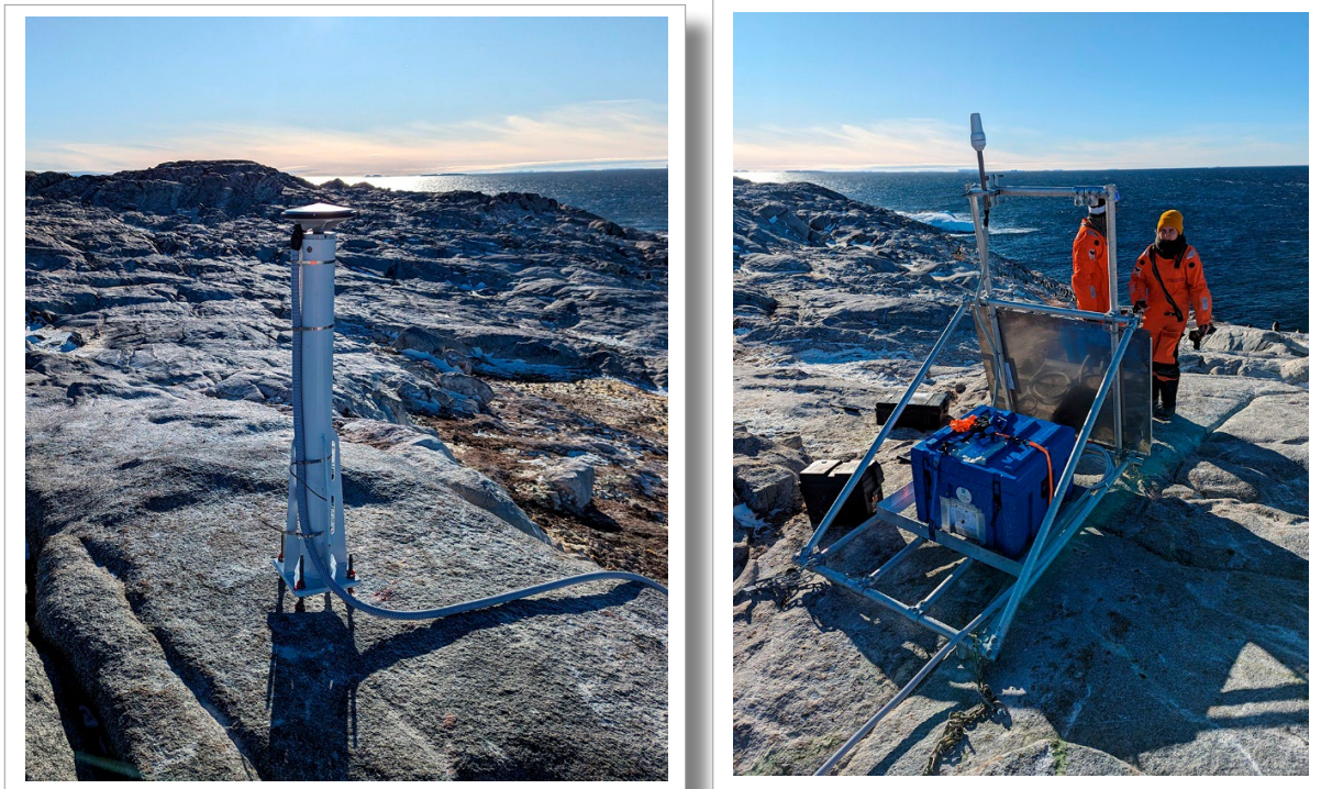
Fig. 6.2.8: (Left) GNSS monument and antenna at IVNF/Ivanhoff Head, looking true west. (Right) New GNSS frame at IVNF/Ivanhoff Head after installation (frame features 160 W solar panel, enclosure with batteries, receiver and Iridium antenna)
