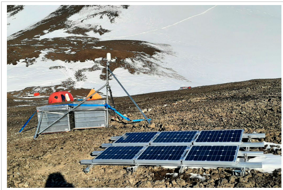
Fig. 6.2.5: GNSS setup at GAP1/Gaussberg, with receiver, Iridium Certus, batteries and further parts contained in the two Zarges aluminium boxes, Iridium antenna on top of the frame, and solar panels installed close to the ground
