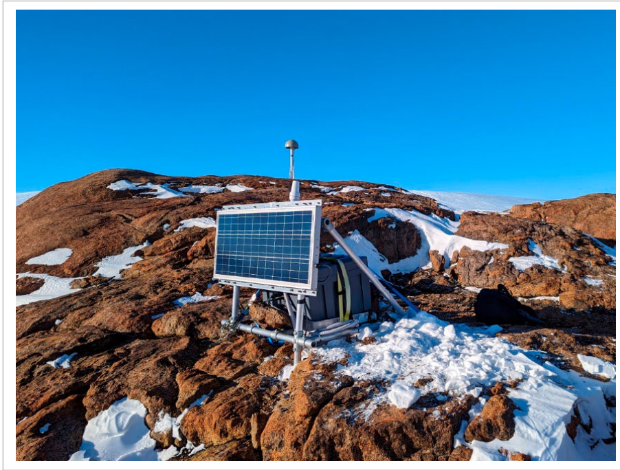
Fig. 6.2.2: GNSS receiver setup at CAD1/Carey Nunatak after upgrade was complete (Iridium antenna installed on frame and enclosure swapped for new GNSS receiver)
