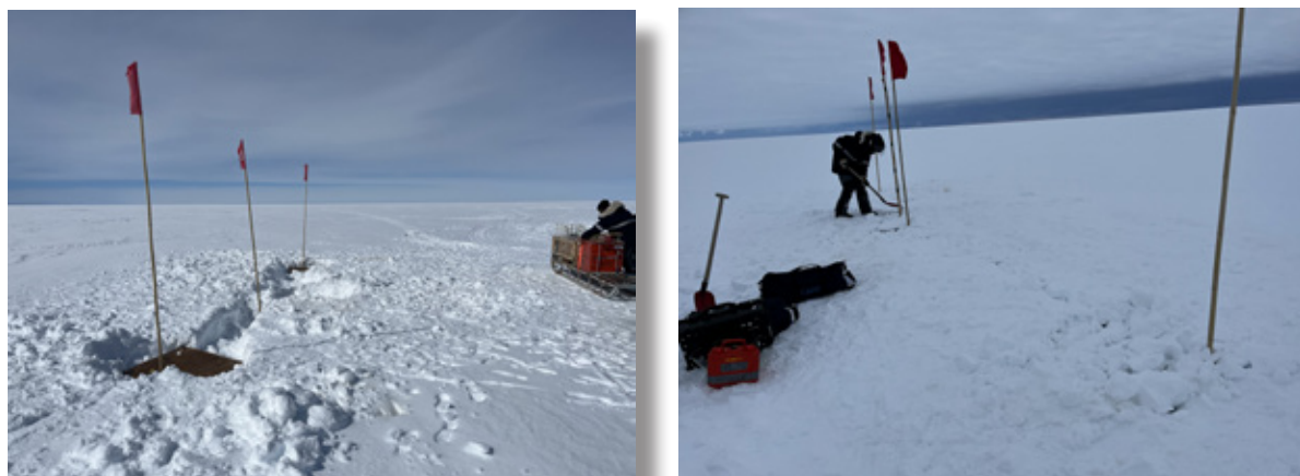
Fig. 4.12.1: Maintenance and new deployment of the ApRES system controller (center pit) and two frame antennas (front and back pits) of the site after completion of the new deployment on 2 January 2023, with the system buried at about 20 cm depth below the current surface (left picture) and system controller (two flags in center) and each frame antenna (left and right flag) covered with wooden boards. The Iridium antenna is mounted on the bamboo pole with black tape (right picture).
