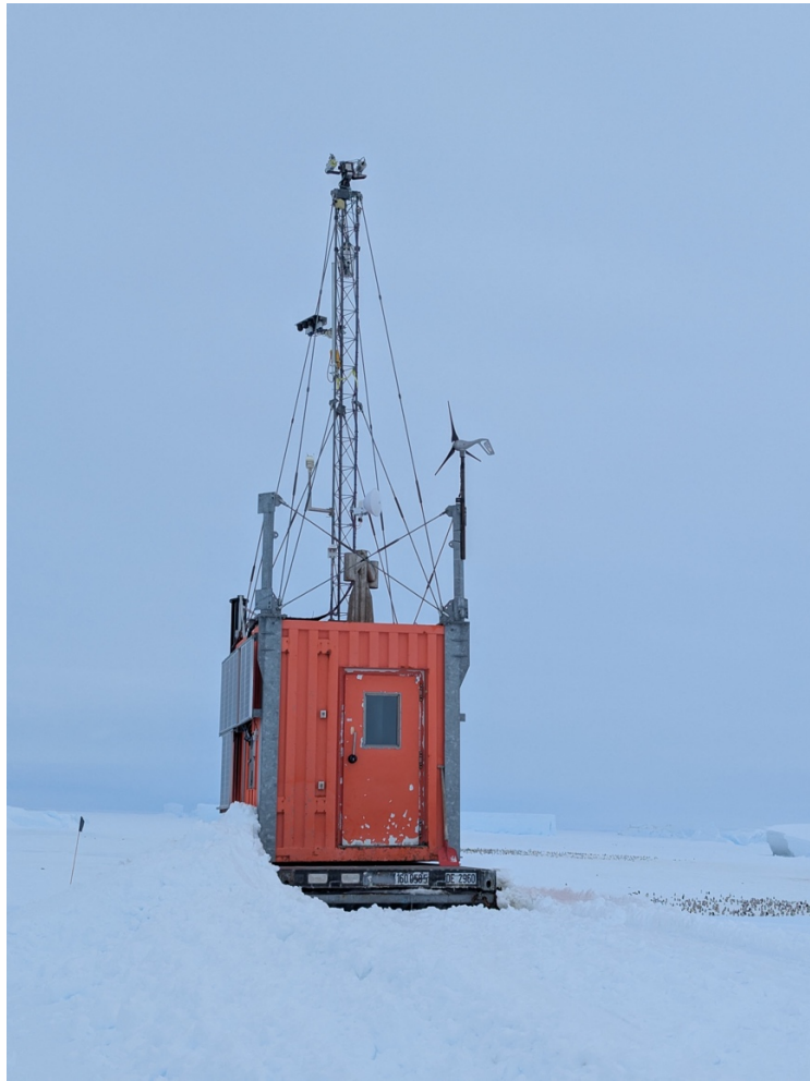
Fig. 4.10.1: SPOT Penguin Observatory in 2025 with new wind turbines
