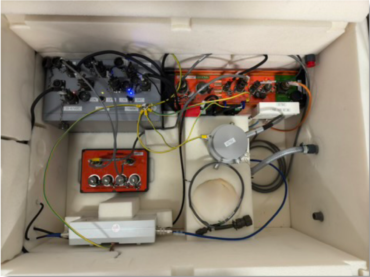
Fig. 4.4.3 The insulated field box contains the microbarometer (centre), the data acquisition system (orange), the power supply (grey) and a communication unit (white). One element is also equipped with a weather station, which is connected to the acquisition system by the red box.
