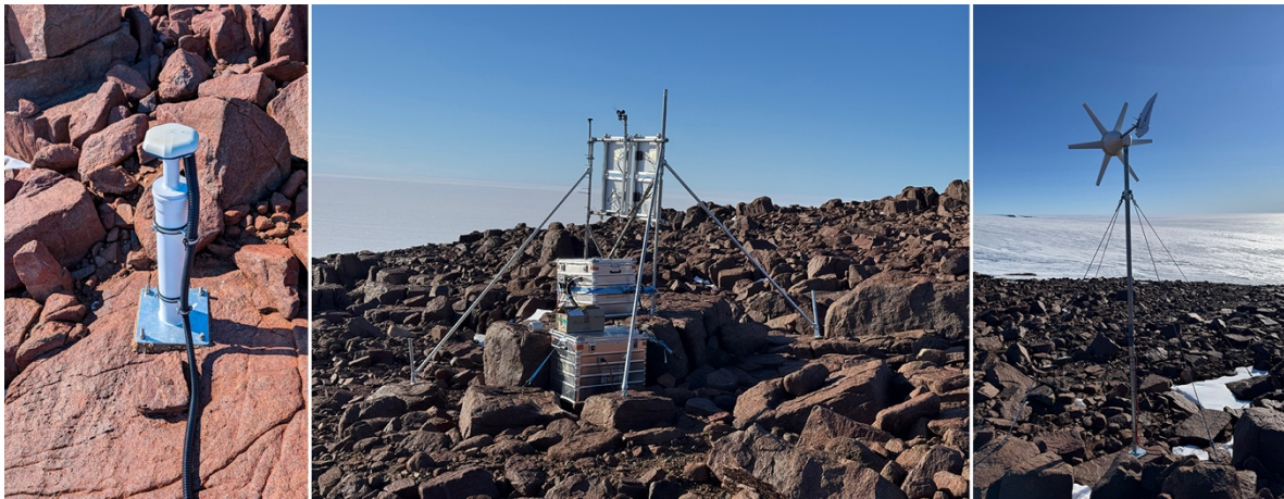
Fig. 4.22.5: GNSS station FOP1 at Forstefjell. Left: GNSS antenna, center: structure with boxes containing GNSS receiver, charge controller, batteries and further electronics, and solar modules; right: wind generator (after it had been repaired).
